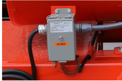
Overnight heating system
